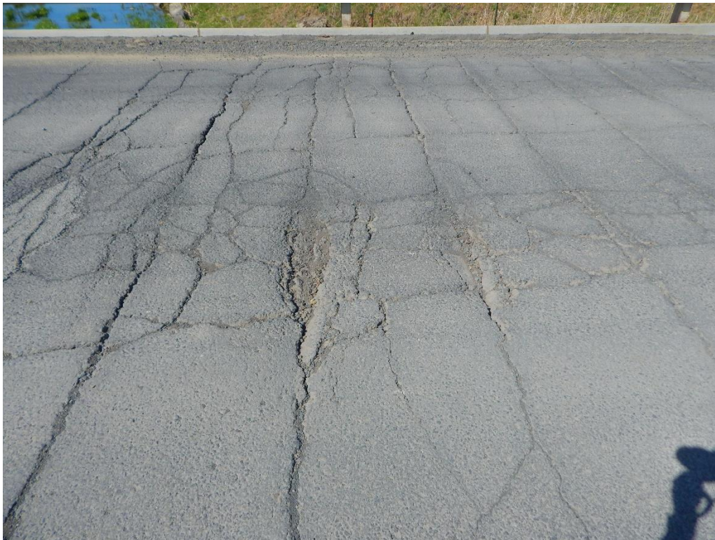
Figure 4 Damaged bridge bed
