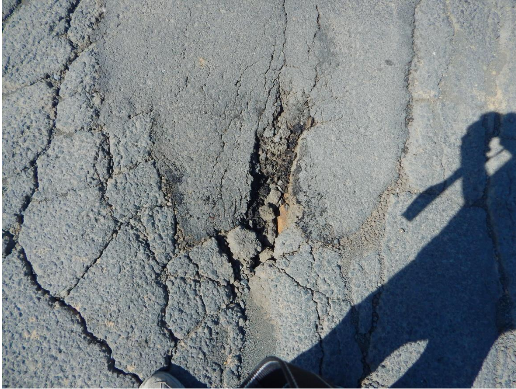
Figure 3 Pothole exposing metal of bridge support
