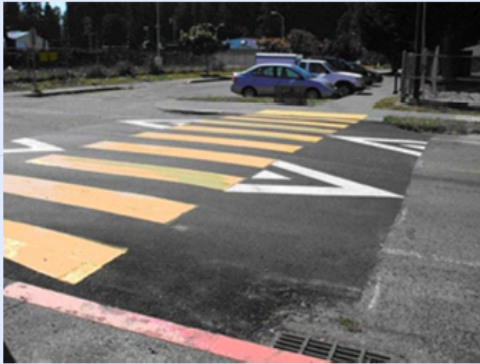
Raised Pedestrian Crossing
