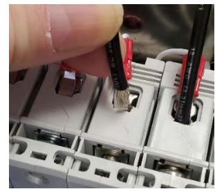
Figure 8 Connecting the load
