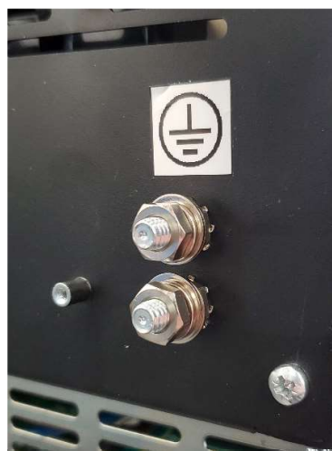
Figure 7A: External Earth Termination
