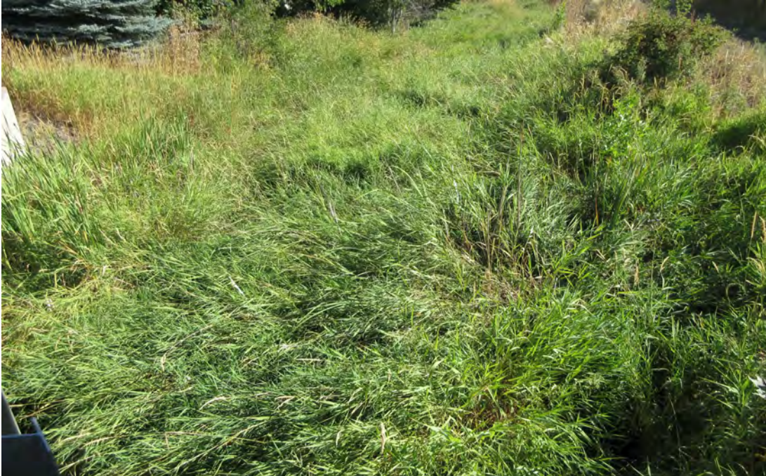
Upstream channel: heavy grass growth is crowding the creek. [Maintenance Recommendation]
