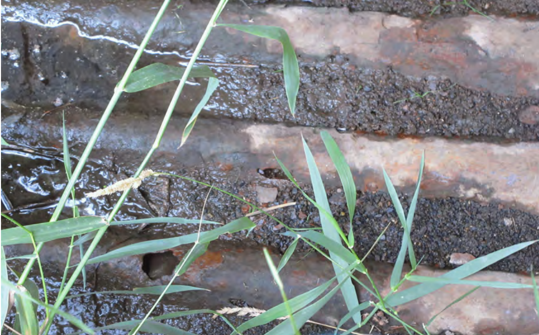
(240-Culvert CS4) South barrel, west end: laminar rust with 100% section loss.
