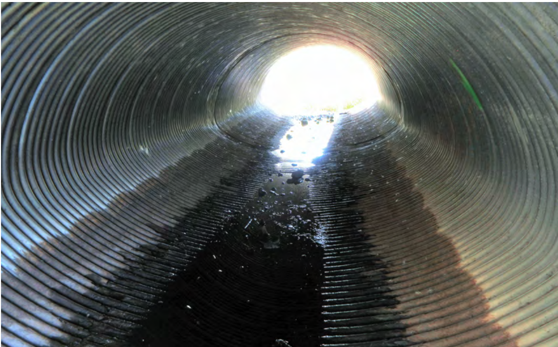
North barrel interior: the base has 100% section loss; the upper coating is in good condition.
