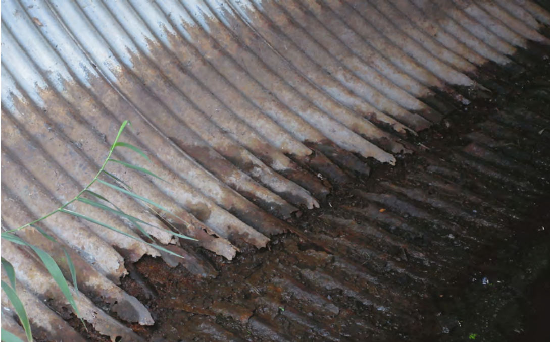
(240-Culvert CS4) North barrel, west end: laminar rust with 100% section loss.
