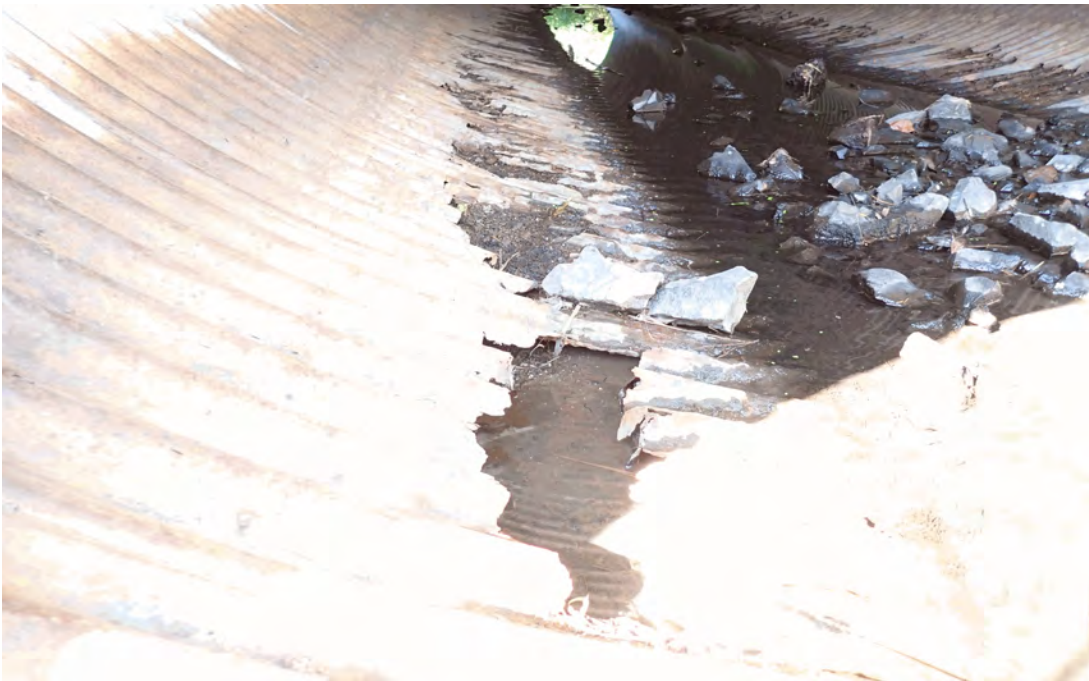
(240-Culvert CS4) North barrel: laminar rust with 100% section loss.
