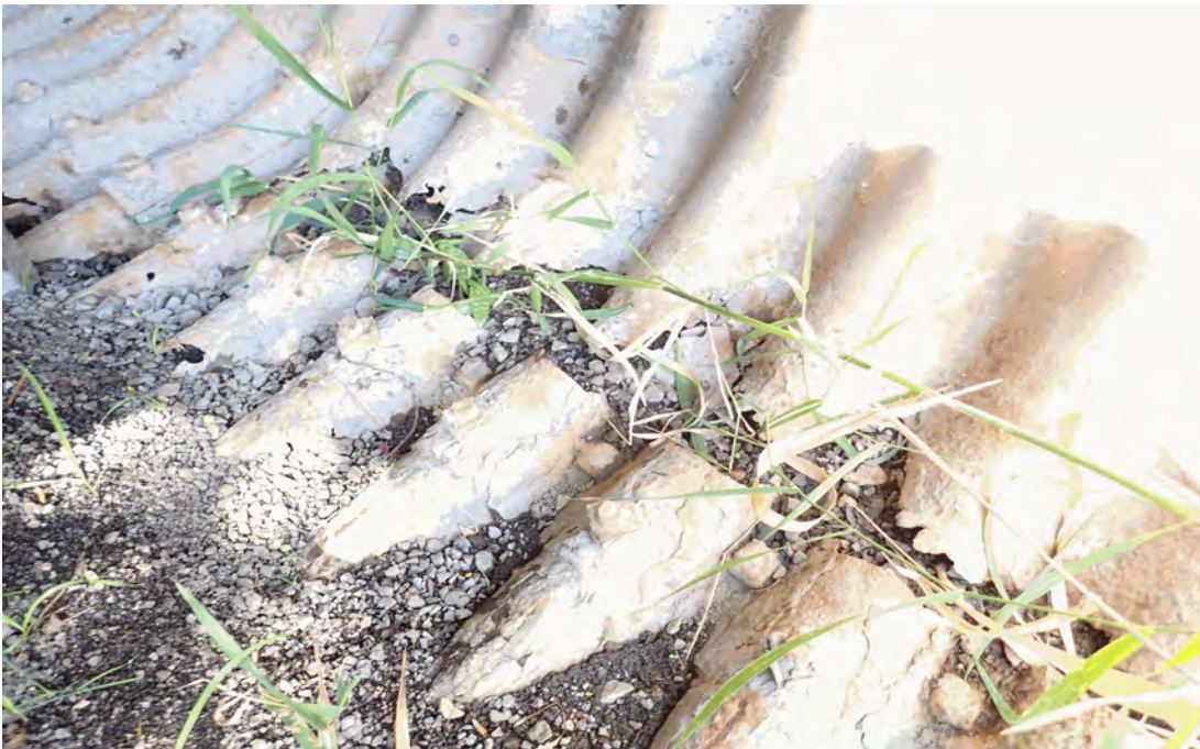
(240-Culvert CS4) South barrel: laminar rust with 100% section loss.
