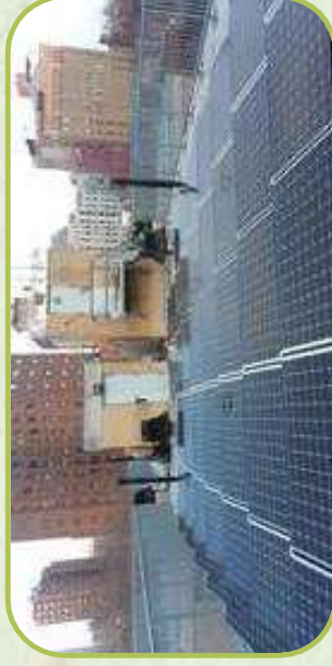
One of several community solar installations on top of NYC Housing Authority buildings
