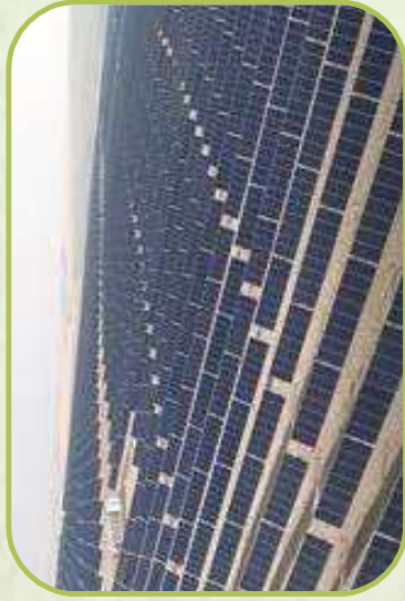
Avista's 200-acre "Solar Select" solar farm for large business subscriptions, located in Lind, WA, owned by Strata Solar
