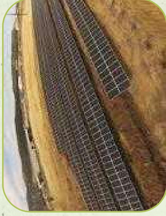
Avista Boulder Park Array
