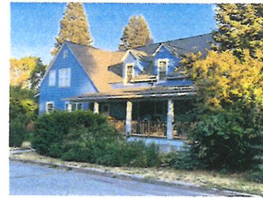
July 2025 Porch Railings
